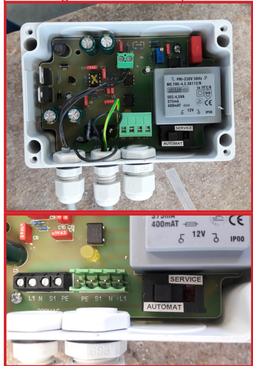
pic. 2: Valve regulator switch
